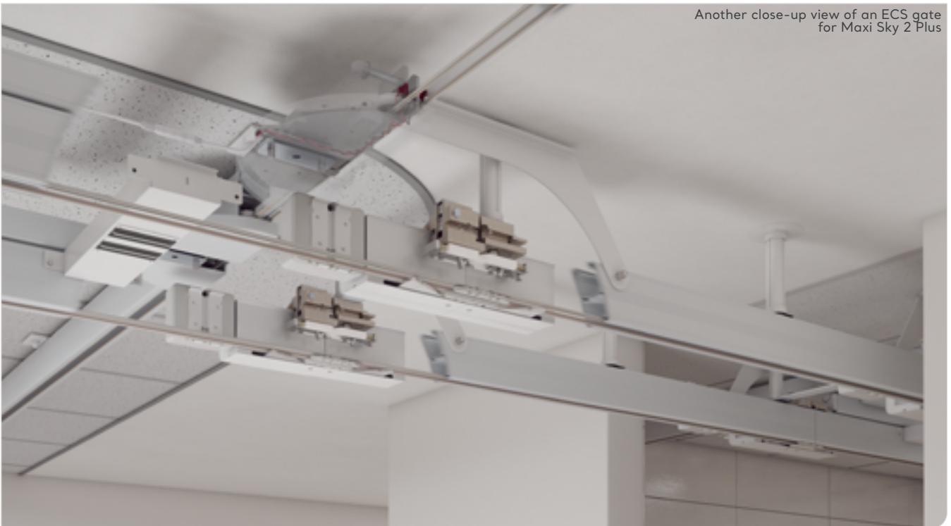
Close-up view of the ECS gate system
